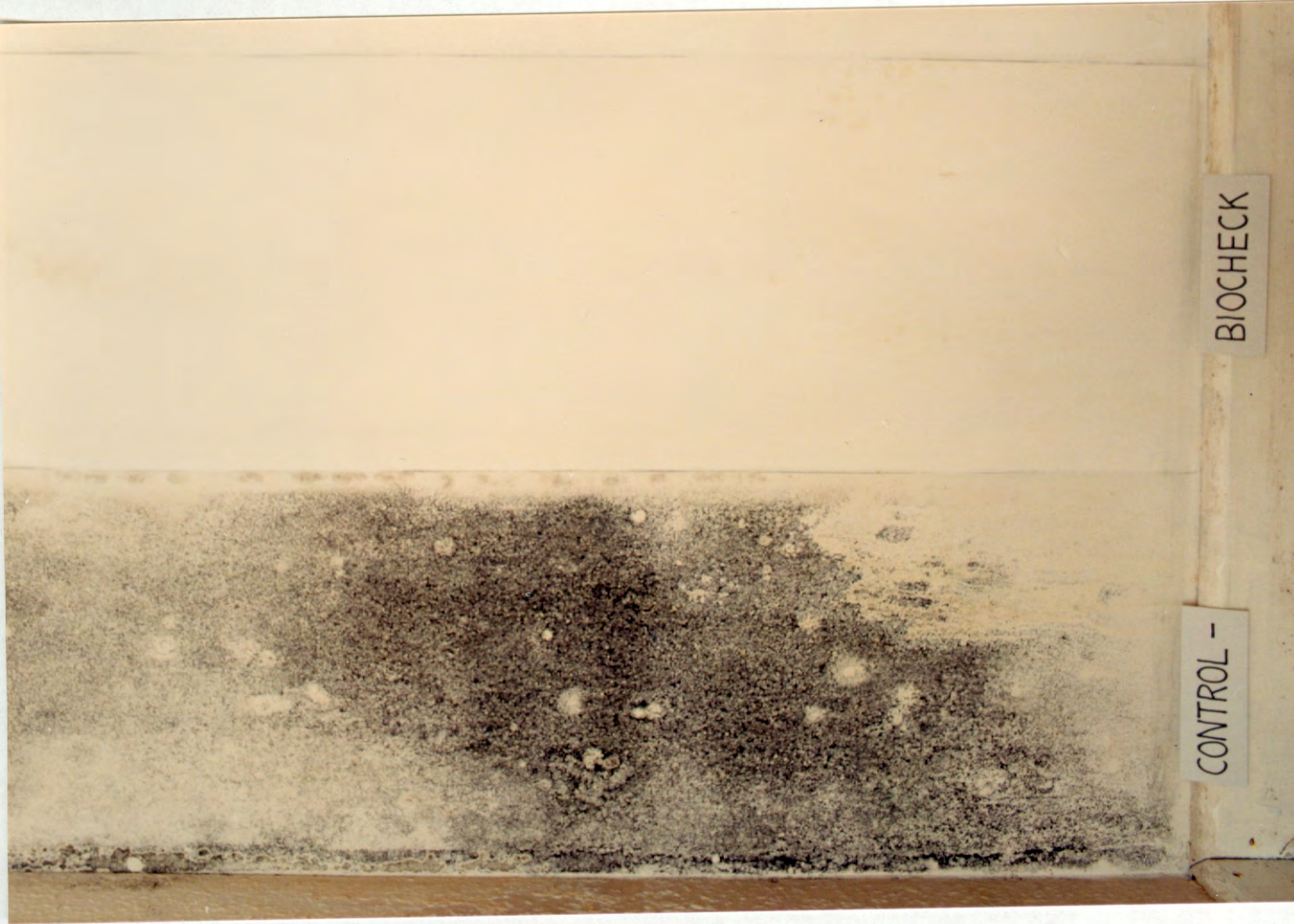
Plate 2 Appearance of paints after 6 months. Neg No 87198.5
