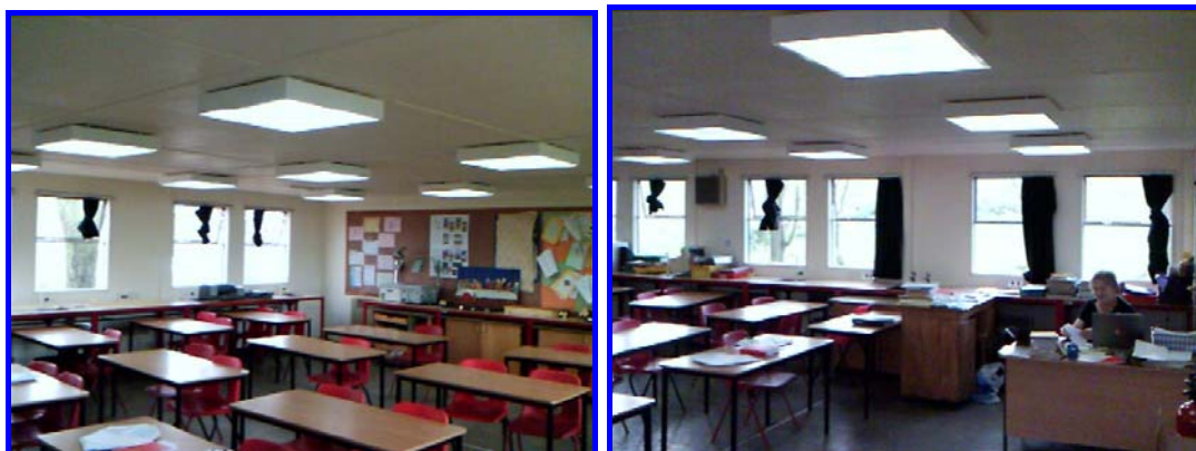
Led Lighting in operation in class room X4 is providing a uniformed level of light.
