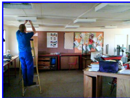
X4 New LED Lighting installed
